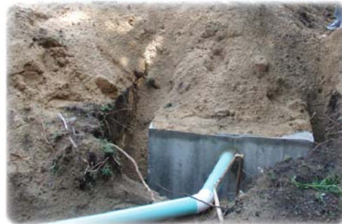
A new septic system was installed to replace the existing failing system.
