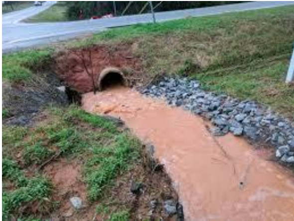
Photo 42 and Photo 43. Examples of issues for Muddy Water Watch
