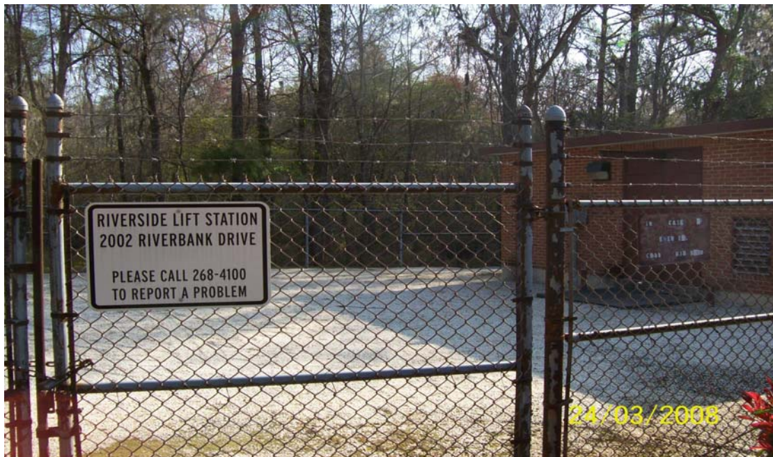
Lift Station located at the banks of impaired station E-105
