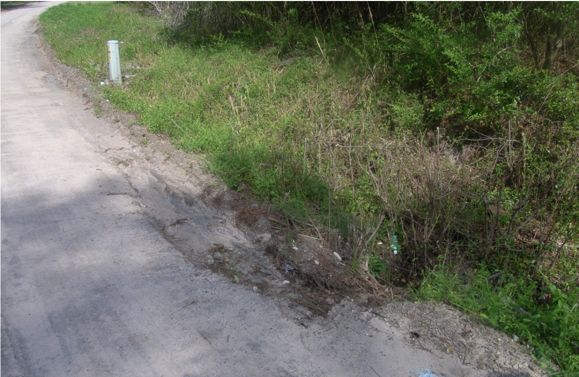
Figure A-9. Erosion of Gravel Road Immediately up-grade of Stream
