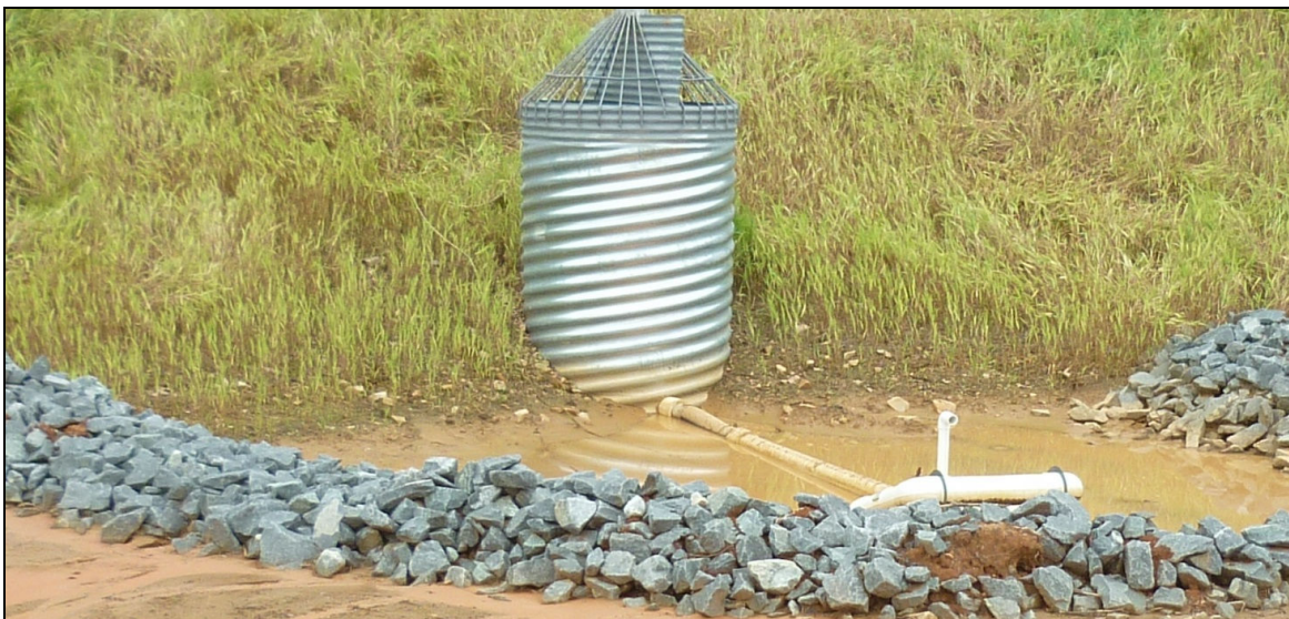
Photo: Principle Spillway's Riser Structure with Skimmer
