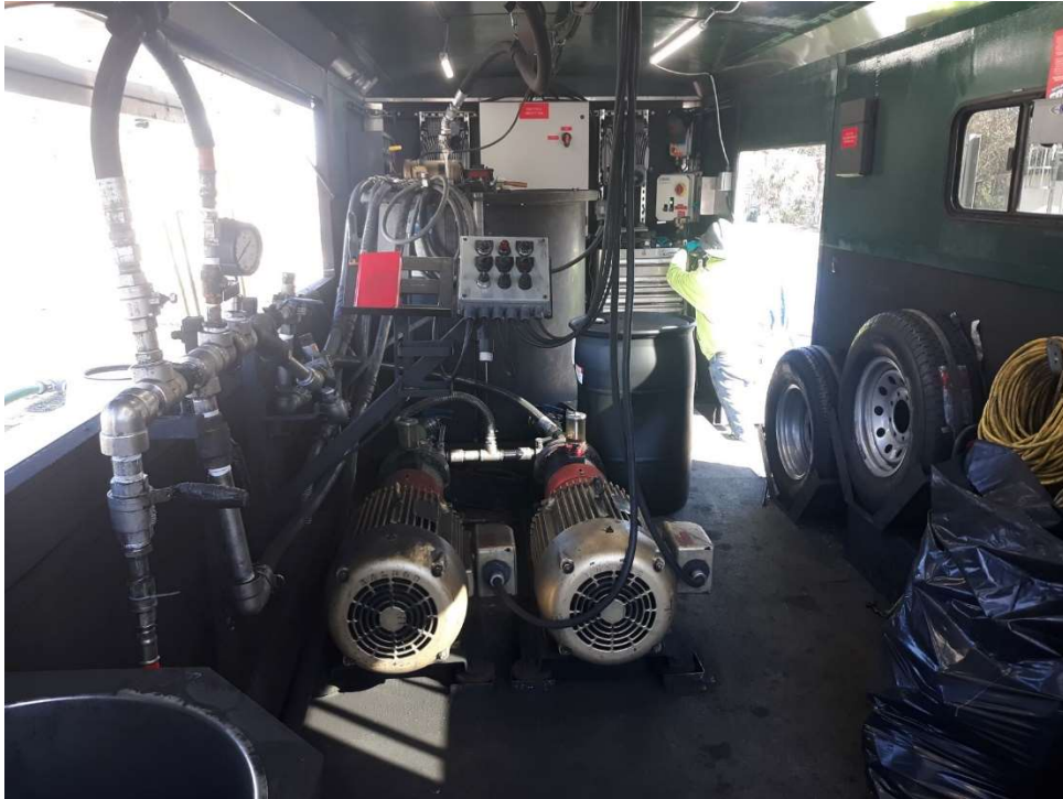
AST injection system (mix tank and pumps) – January 19, 2022
