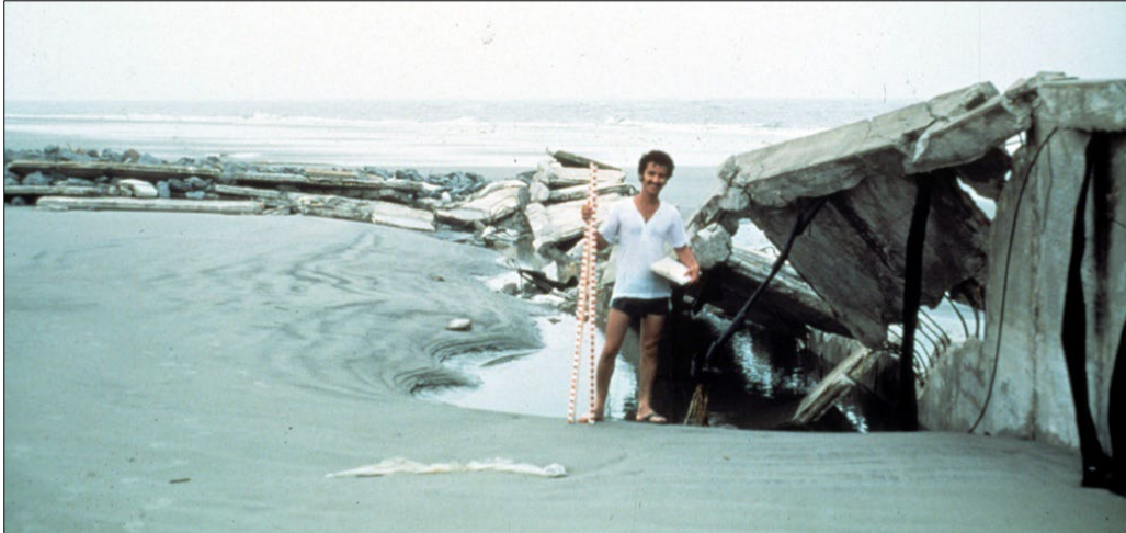
FIGURE 3.4. Concrete sheet pile seawalls were installed along portions of reaches 5 and 6 in the 1970s. As they became more exposed, rip rap and larger armor stone was added for reinforcement and scour protection. Image shows a section of the concrete seawall after a collapse during Hurricane David (September 1979). [Source photo by Research Planning Institute Inc.]
