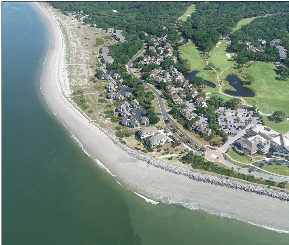
FIGURE 3.6. Section of exposed seawall in the critically eroded Reach 3 on 15 May 2020. The crest elevation of the wall is lower and the armor stone is smaller in front of the homes in the image. This is considered the most vulnerable section of the beach at present. [Photo by J. Hair – CSE]
