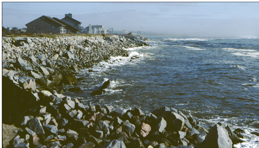
FIGURE 3.2. Beach erosion in reaches 6 and 7 (see Fig 1.1) led to exposed seawalls, no recreational beach, and severe damage to structures in 1983. View north along Reach 7 in 1985 at low tide. [After CSE 1989]
