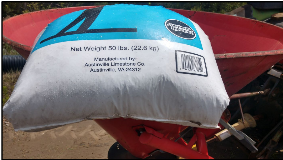
Photo 2: View of packaged Lime that was applied to GP Mine area side slopes and surface water perimeter (04/20/20).
